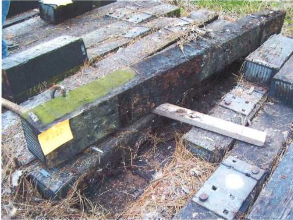
Figure 57 - Tie #260 (Koppers/red oak/creosote petroleum).
