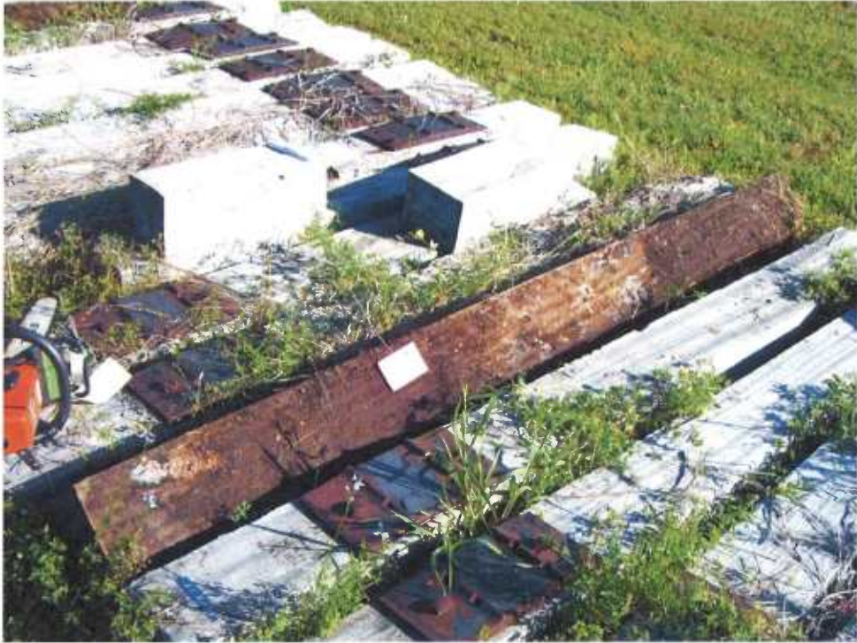
Figure 1 - Tie #8 (Turada) with light decay.
