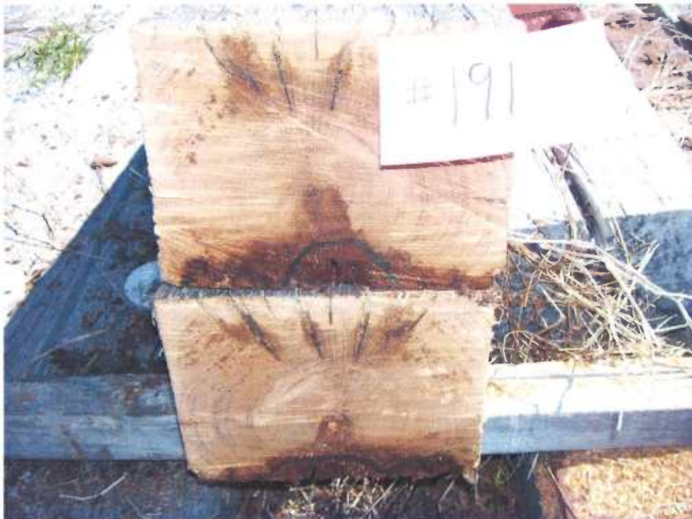
Figure 42 - Tie #191 (Cedarcide/white oak) with decay.
