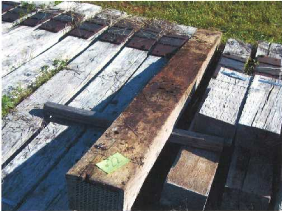
Figure 5 – Tie #22 (Envirosafe/white oak) with light decay on bottom.
