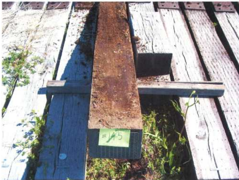
Figure 29 - Tie #145 (Lonza/White oak) with decay on bottom.
