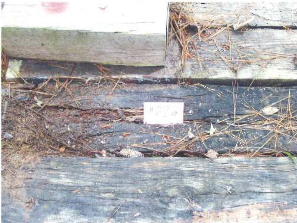
Figure 4 - Tie #226 (red oak/control) with heavy decay.
