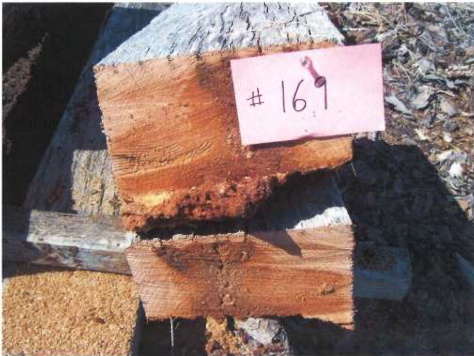
Figure 36 - Tie #169 (red oak control) failed due to decay.
