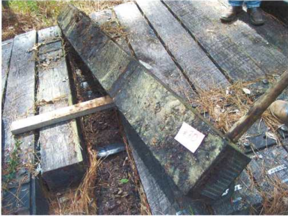
Figure 13- Tie#70 (Boatright/red oak/creosote 5pcf).
