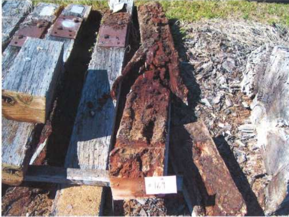
Figure 35 Tie #169 (red oak control) decayed to the point of failure.
