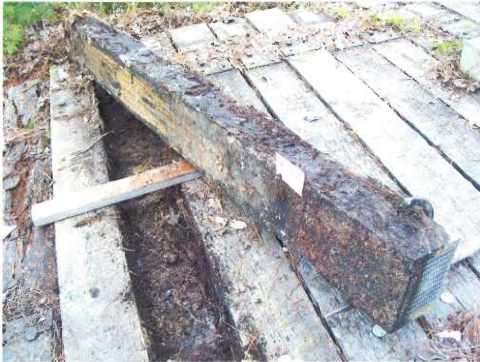
Figure 21- Tie #113 (Lonza/white oak) with trace decay mycelium growing.
