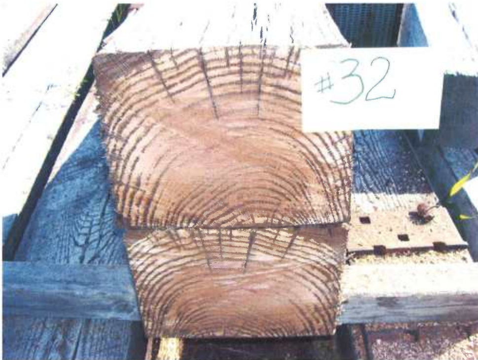
Figure 8 – Tie #32 (Boatright/red oak/creosote 5pcf).
