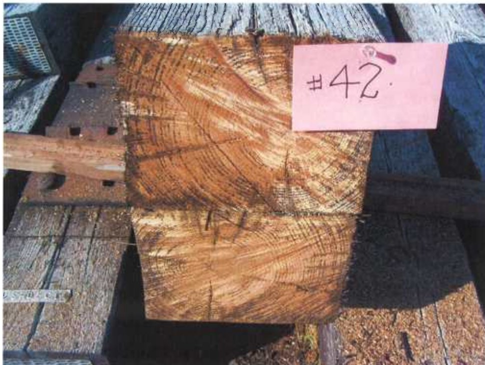
Figure 10 - Tie #42 (Boatright/red oak/borate/creosote 5pcf).
