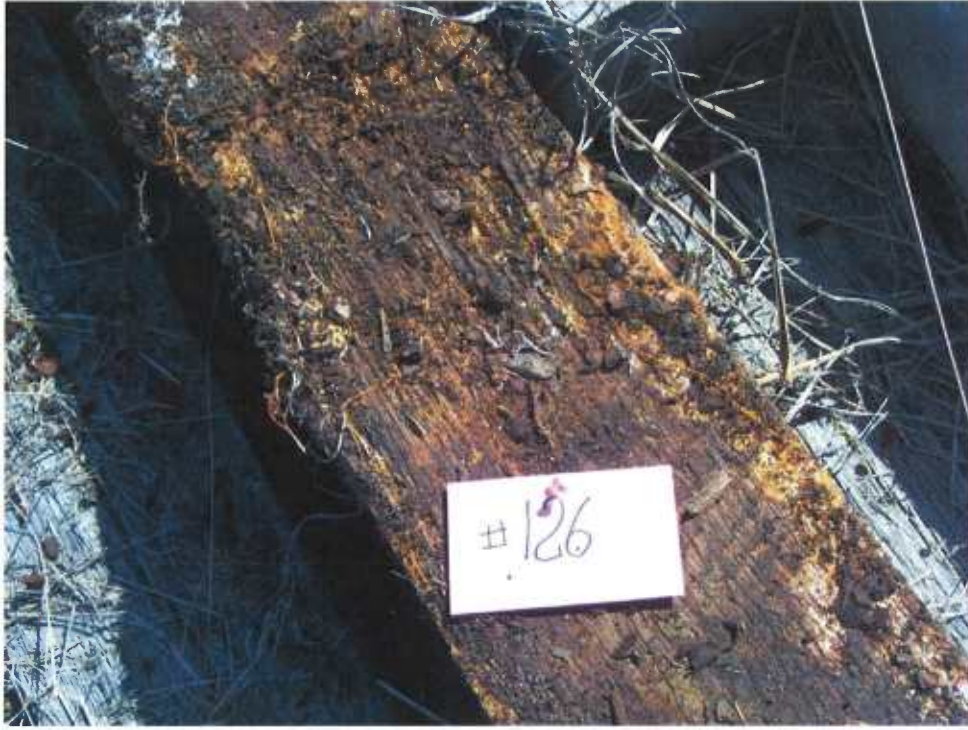
Figure 5 - Tie #126 with decay on bottom surface.
