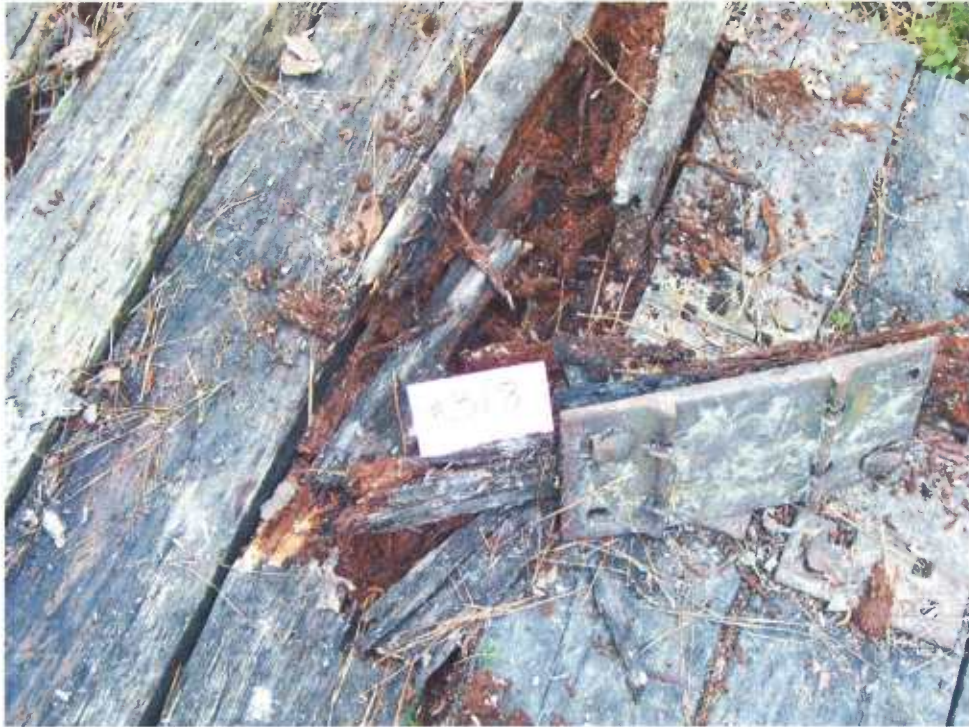
Figure 3 - Tie #318 (red oak/control) showing severe decay damage.
