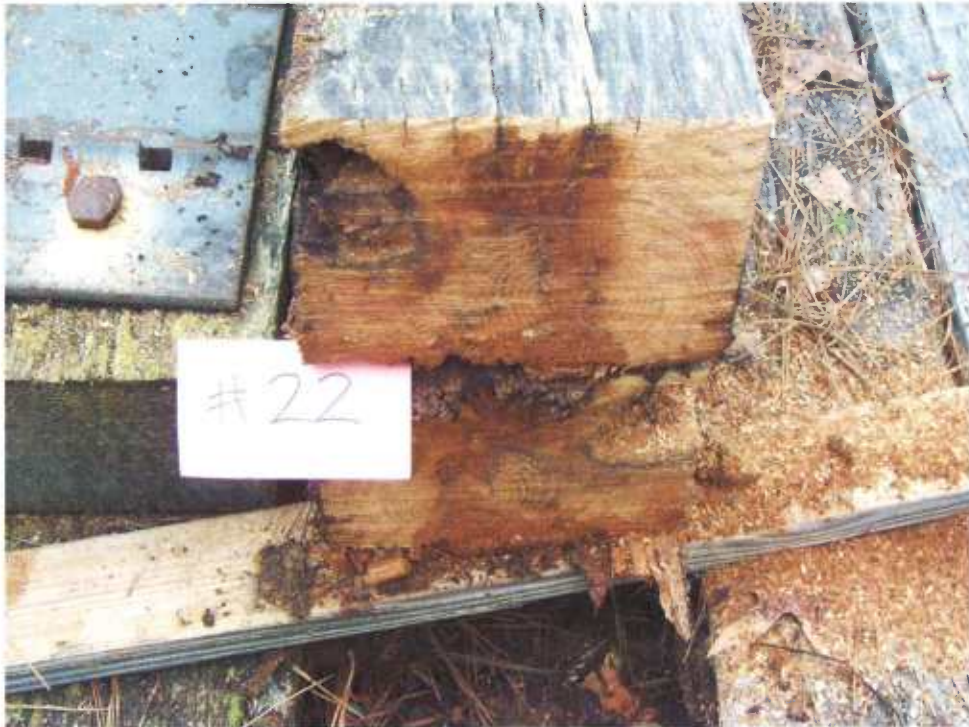
Figure 4- Tie #22 (Cedar/cide/red oak) showing areas of decay.
