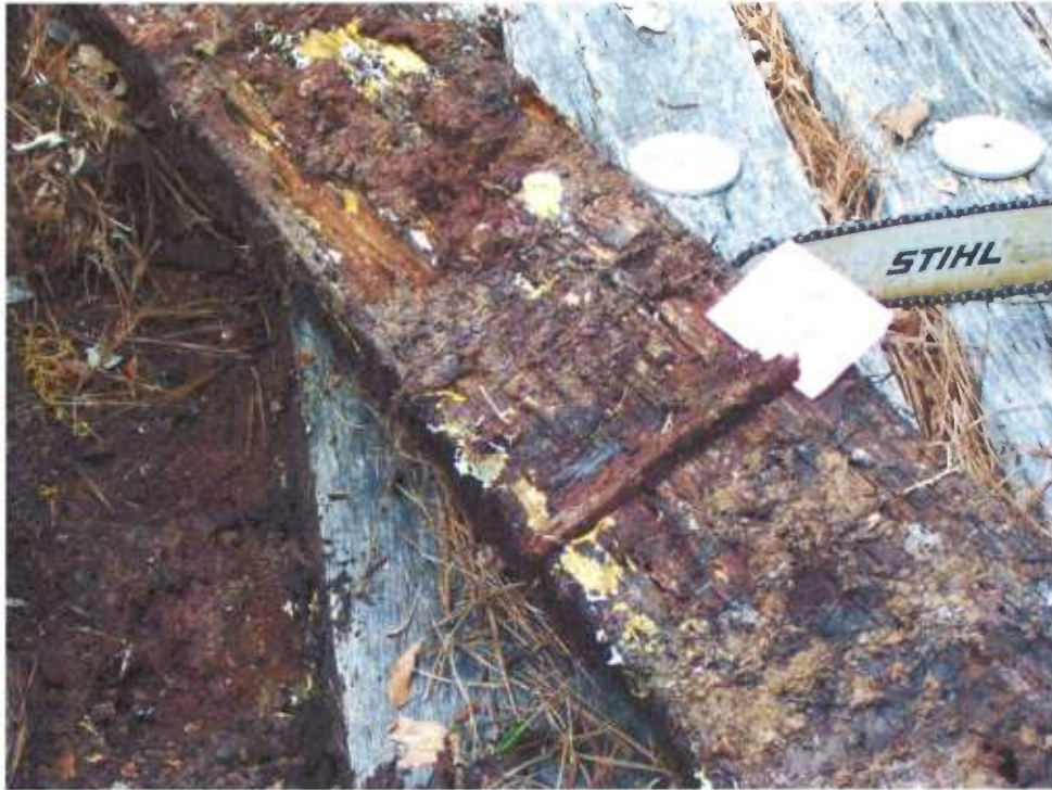
Figure 3 - Tie #22 (Cedarcide/red oak) with decay and beetle damage.
