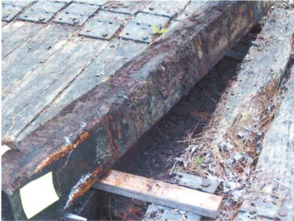
Figure 61 - Tie #322 (Envirosafe/white oak) with termite grazing and trace decay.
