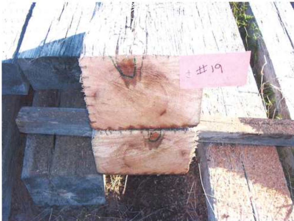
Figure 4 – Tie #19 (Envirosafe/red oak) with decay around check.
