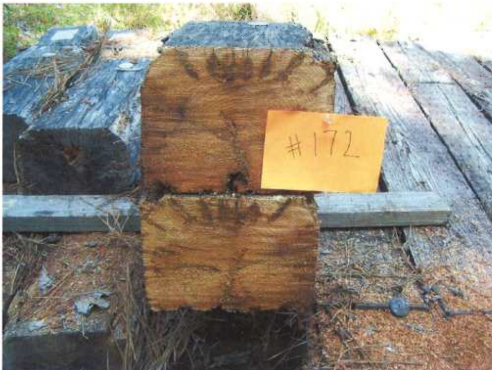
Figure 36 - Tie #172 (red oak/control) with decay visible in cross-section.
