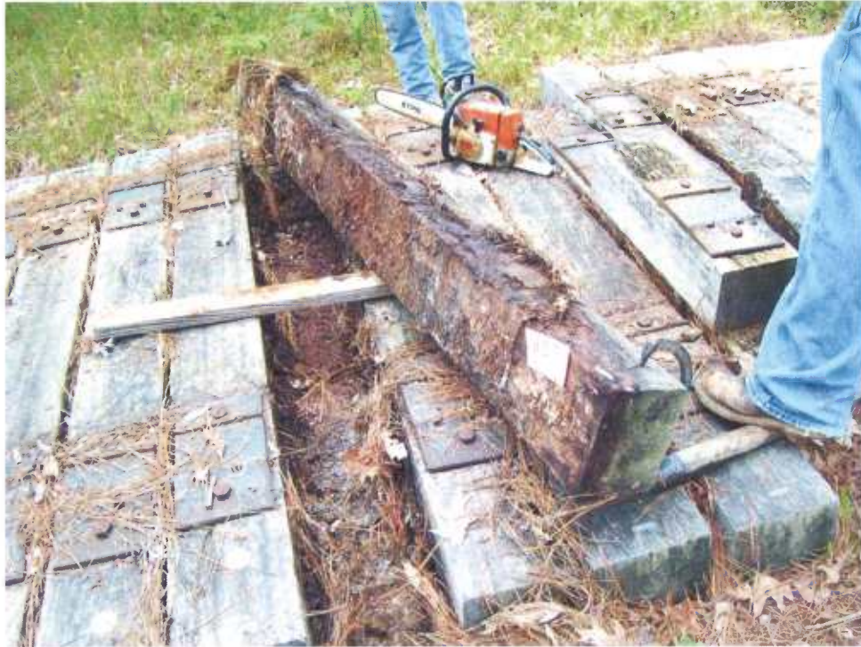
Figure 5 - Tie #27 (Turada) with trace decay.
