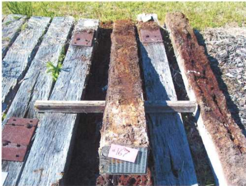
Figure 33 - Tie #167 (white oak control) with decay evident on all surfaces.
