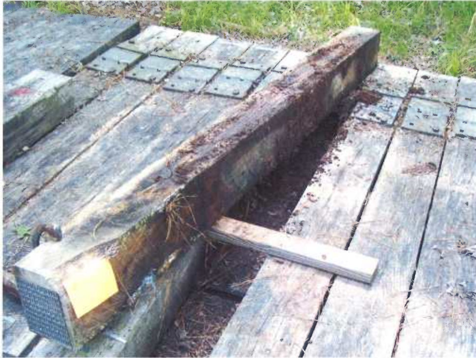
Figure 59 - Tie #290 (Envirosafe/red oak) termite surface etching and trace decay.
