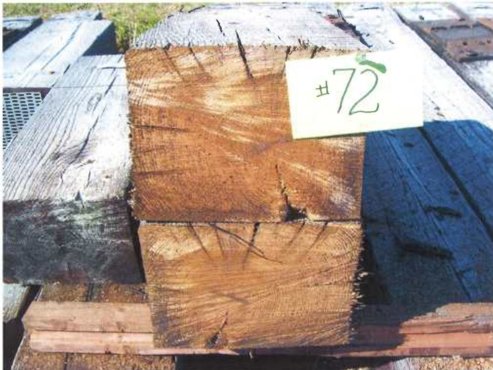
Figure 16 - Tie #72 (Boatright/red oak/borate/creosote 7pcf) knot hole/pocket on bottom.
