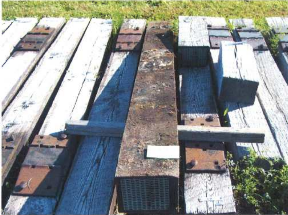
Figure 7 – Tie #32 (Boatright/red oak/creosote 5pcf).
