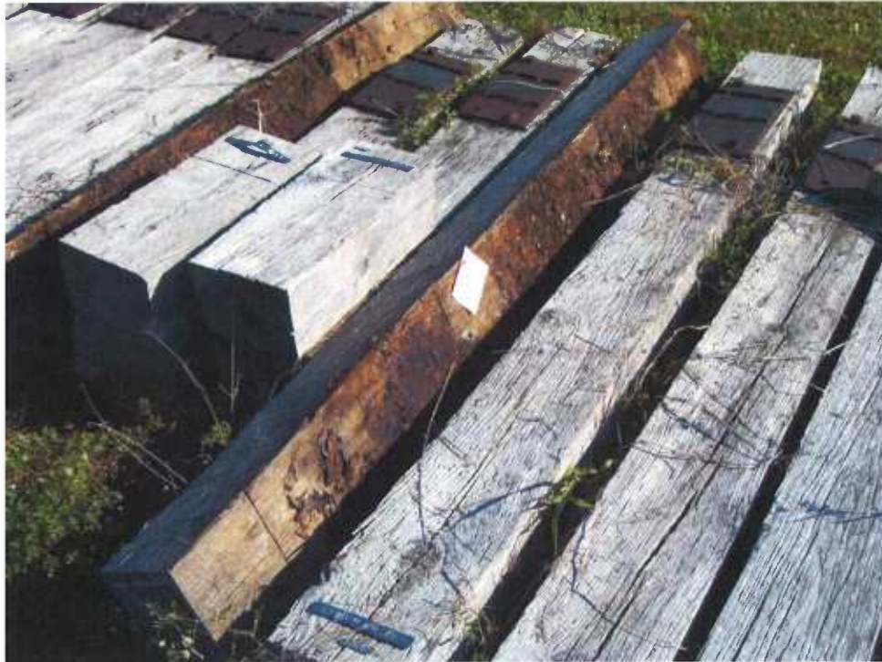
Figure 3 – Tie #19 (Envirosafe/red oak) with light decay.
